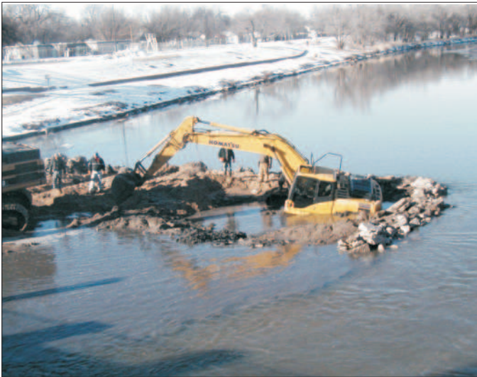
A backhoe gets swamped during construction of the temporary footbridge across the river near North High.
